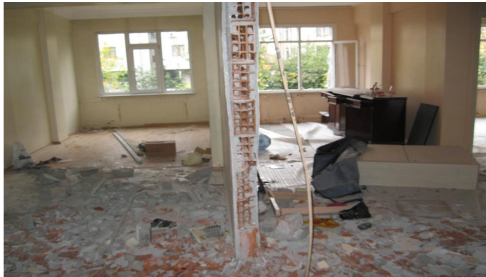
Figure 3.15 : Crushing of inner walls of the building.
