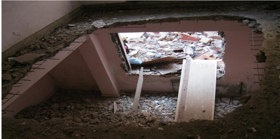
Figure 3.9 : Accumulation of debris at the basement.
