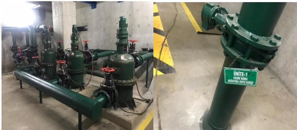
Figure 4.4. Penstock and Butterfly Valves.
