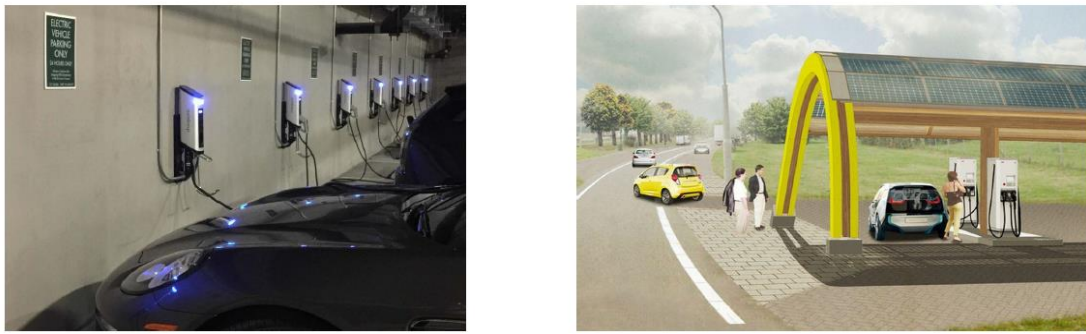
Figure 3.6. Dependent and independent charging stations.
