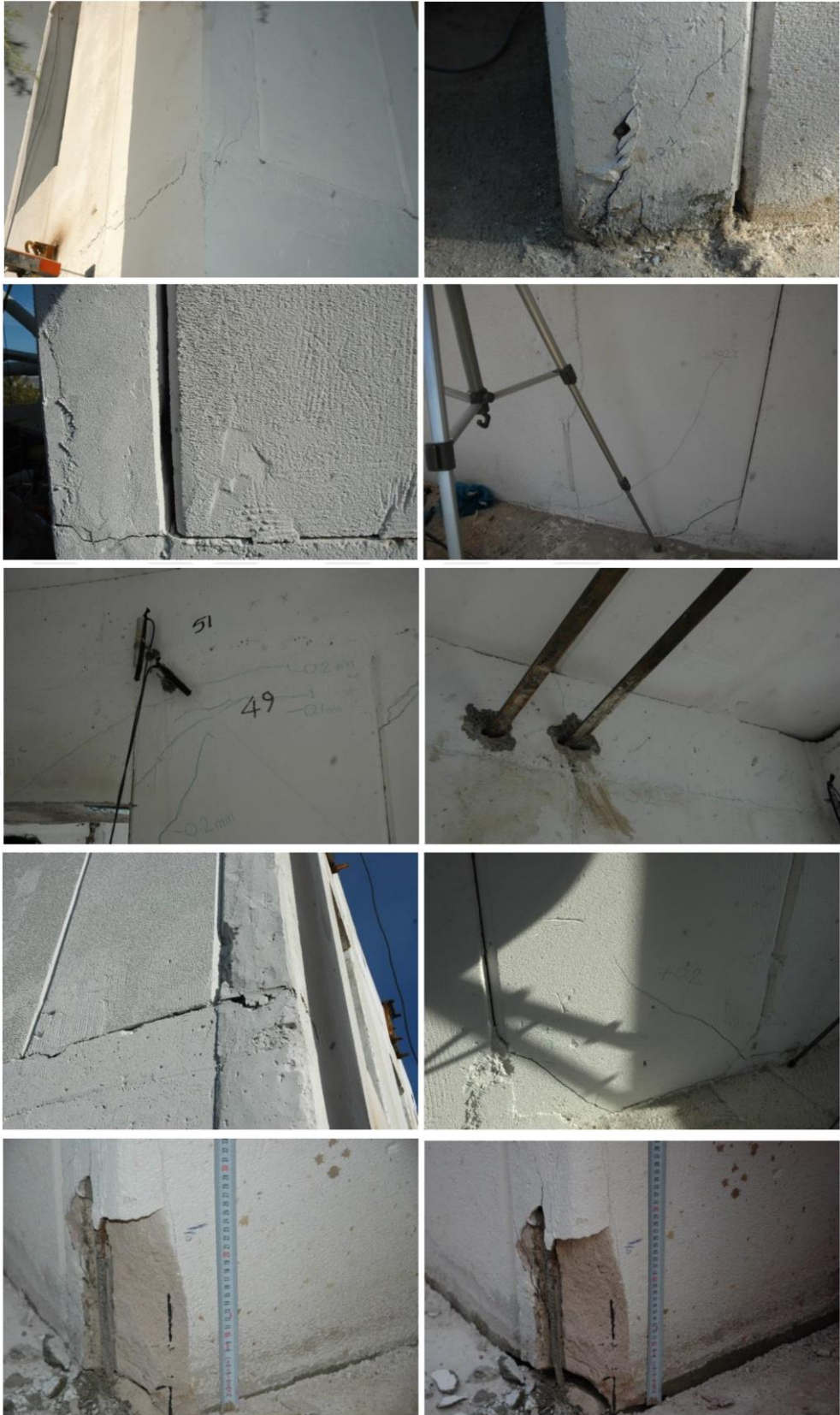
Figure 2.16: Damage Pictures of Project Building
