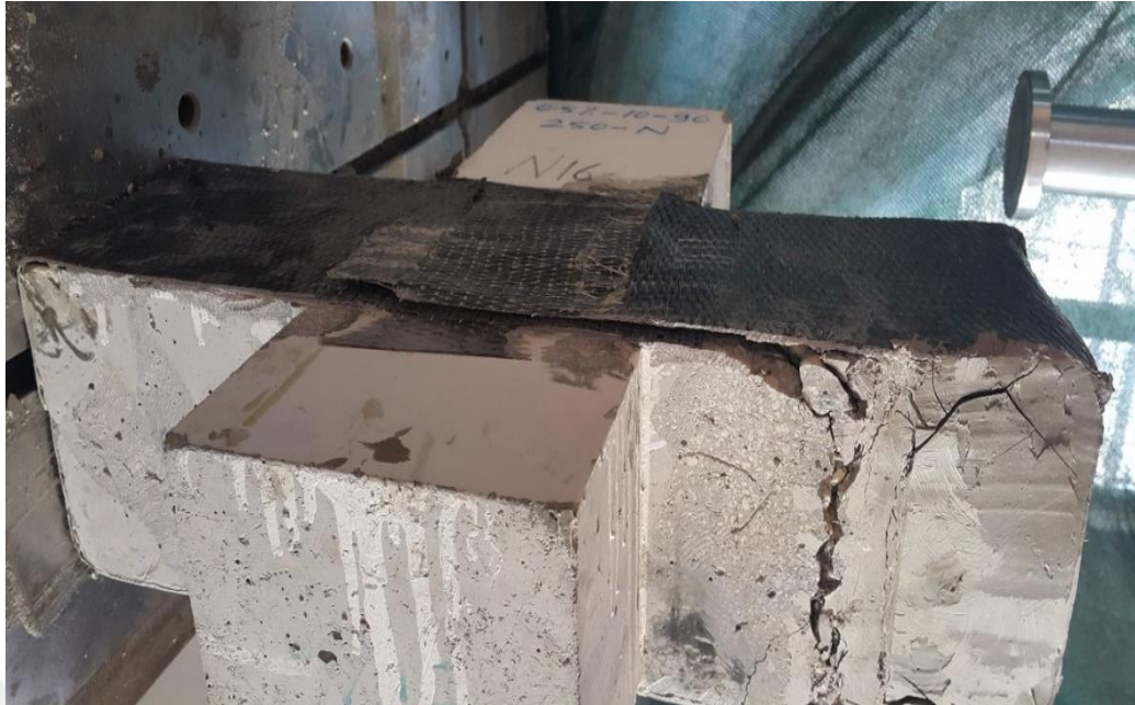
Figure 4.39 Specimen (C13-0.5-250) de-bonding failure after strengthening C14-0.5-500:
