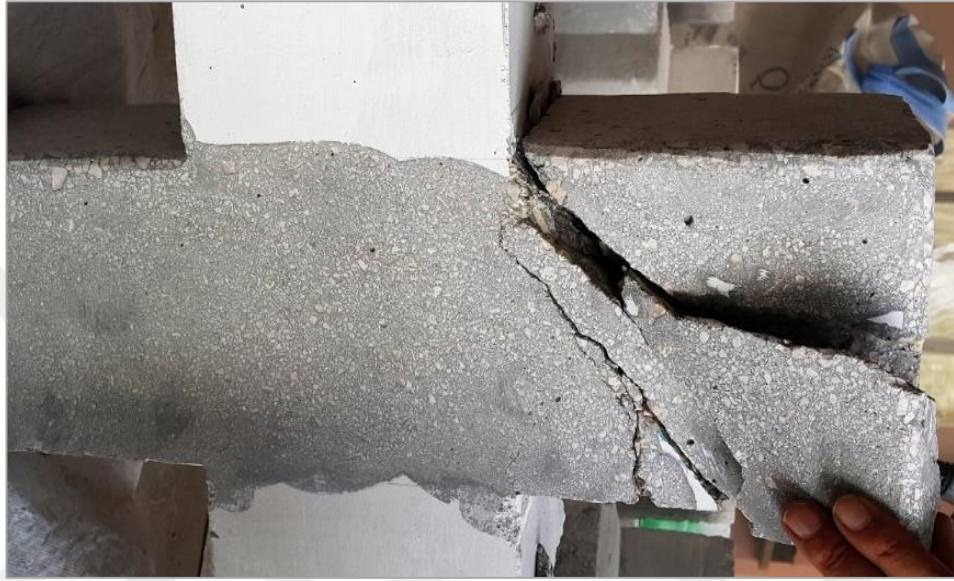
Figure 3.3 High damaged corbel
