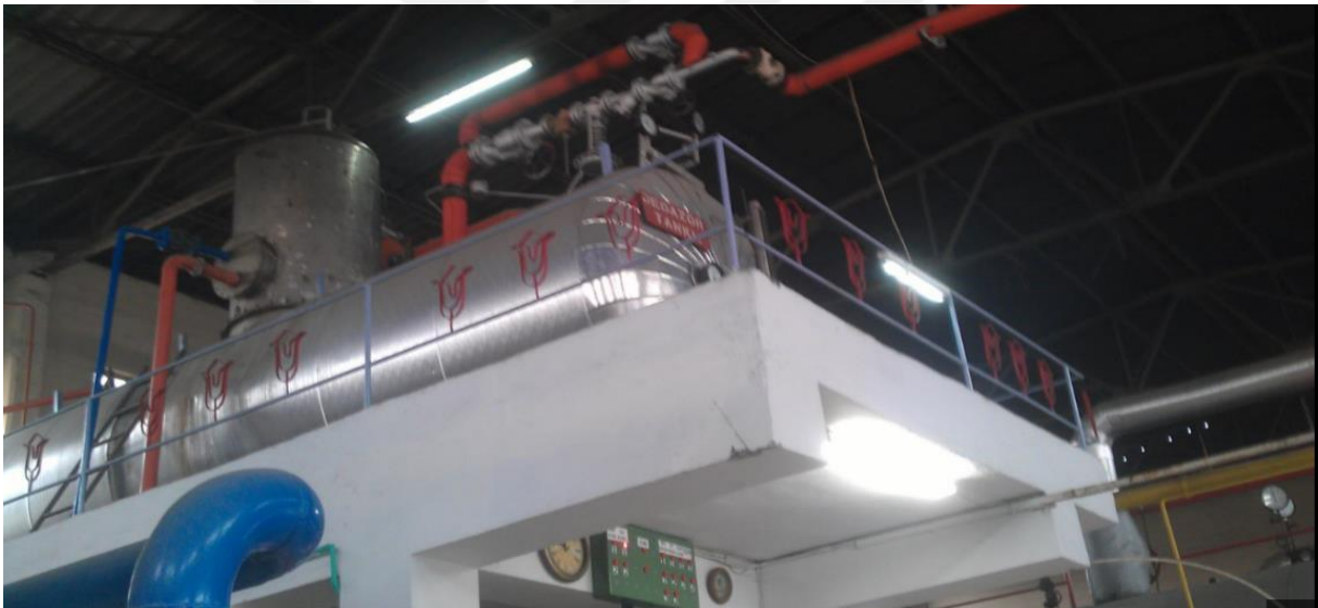
Figure 6.15 Degasifier (photo taken by the author)
