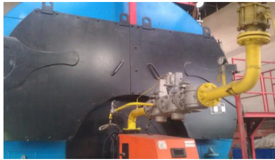
Figure 6.17 Hot water boiler (photo taken by the author)
