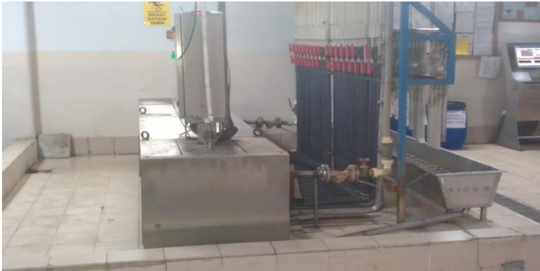
Figure 6.8 Chemical distribution area (photo taken by the author)
