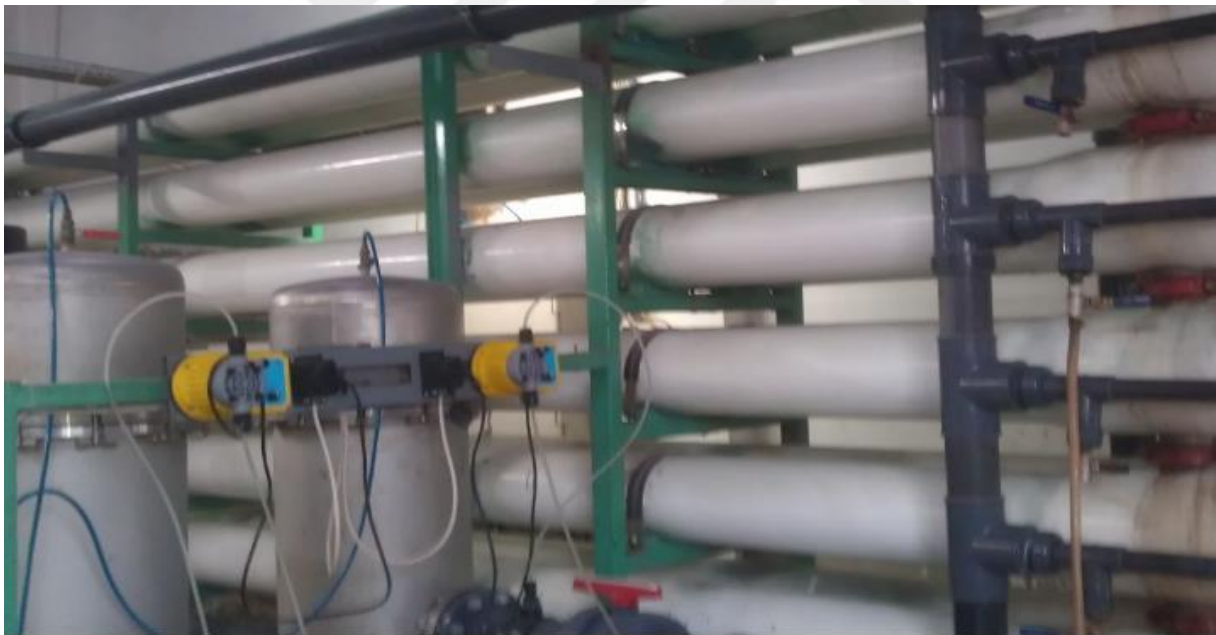
Figure 6.21 Membrane technology-Reverse osmosis (photo taken by the author)
