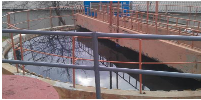
Figure 6.20 Sedimentation (photo taken by the author)
