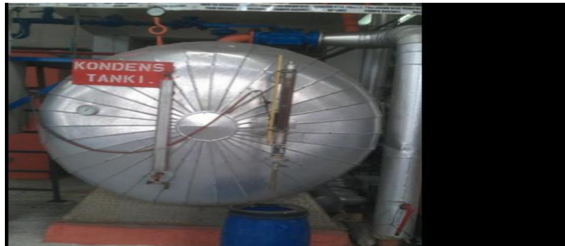
Figure 6.16 Condensate tank (photo taken by the author)
