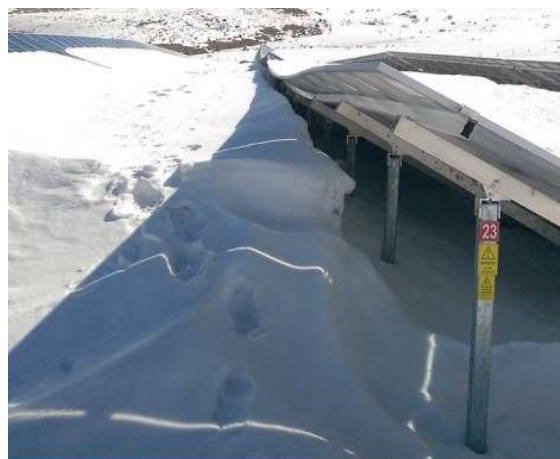
Figure 36- Snow Accumulation on PV Panels-3
