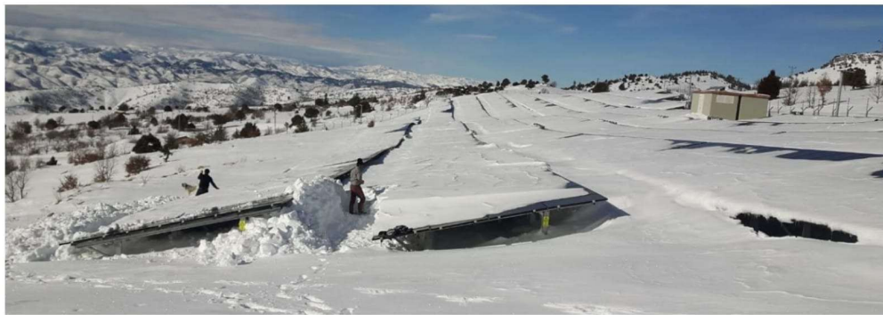
Figure 35- Snow Accumulation on PV Panels-2
