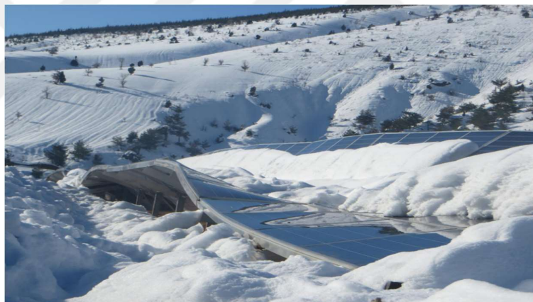
Figure 3- Damaged PV Mounting Structures, Ekol Loss Adjusting (2018)
