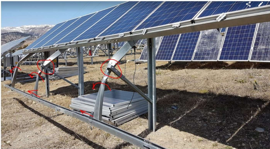
Figure 37- Damaged Main Beam-1
