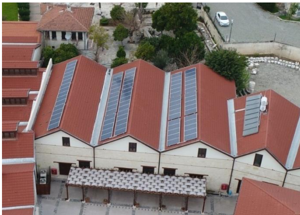
Figure 46. Photovoltaic and Solar Panels of the building for heating and hot water, on the roof of Building B and C(Source: SAYKA, 2025)
