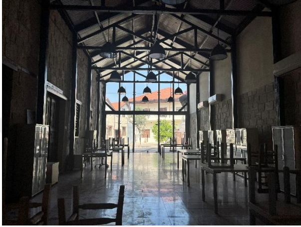
Figure 52. Poor daylighting of open work area from the entrance of Building A from Abdi İpekçi Street.
