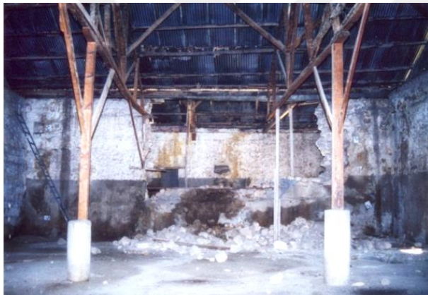
Figure 34. Deformations on the existing walls (SAYKA,2025)
