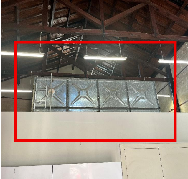
Figure 28. Rainwater Storage Tank in Building C is located in Security room which is the room next to the library
