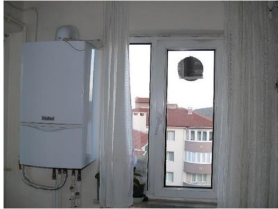
Figure 4. The combi boiler installed on the interior wall of the kitchen, with a window vent covered with paper (Akgün, 2019).
