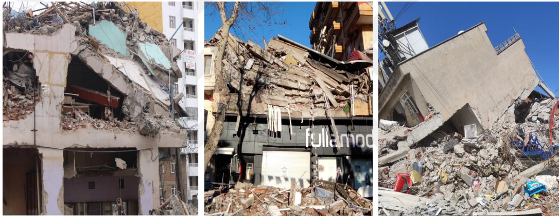
Figure 5.27 : Examples of damage due to strong beam-weak columns
