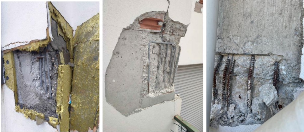
Figure 5.25 : Field observation of inadequate reinforcement and inferior construction practice
