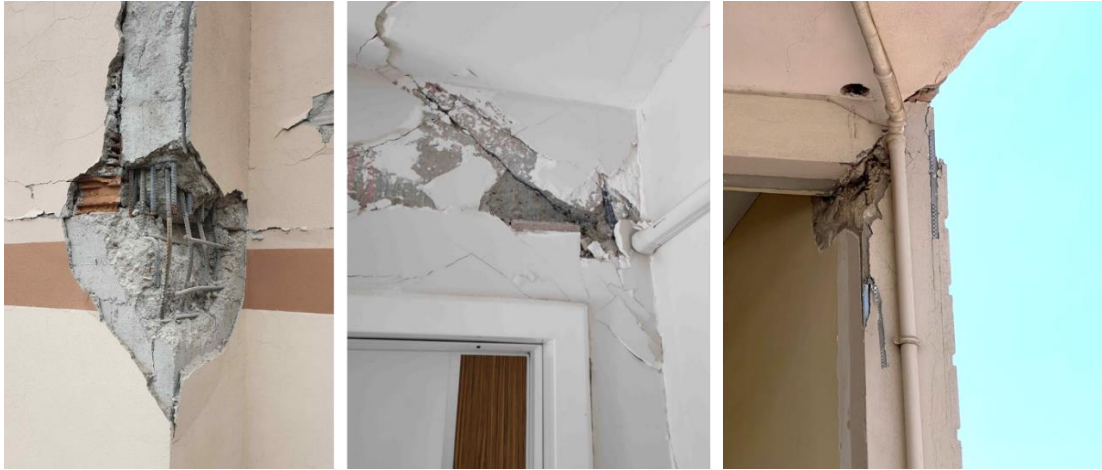
Figure 5.24 : Field observations of damaged RC members showing beam-column joint failures
