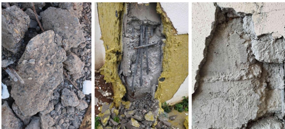
Figure 5.26 : Substandard practices, such as oversized aggregates and poor bonding.
