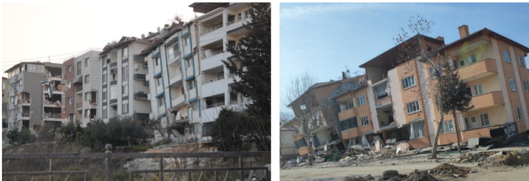
Figure 5.1 : Damage due to pounding effect
