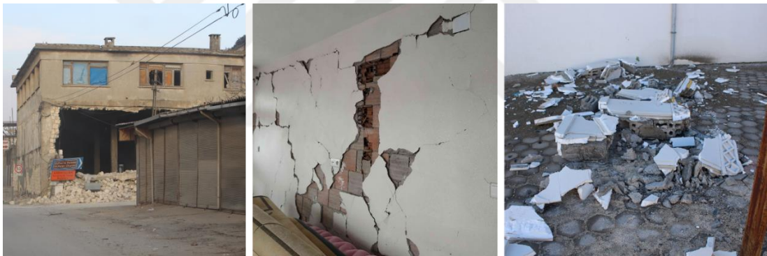
Figure 5.2 : Field evidence of nonstructural damage
