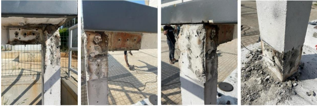
Figure 5.23 : Post-test examination of the beam–column connection of Specimen 2 after 1 g Kahramanmaraş earthquake following removal of the anchor plates, showing localized concrete spalling and embedded steel plate details.
