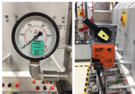
Figure 5.2. Manometer and Electrical Valve on the Test Bench
