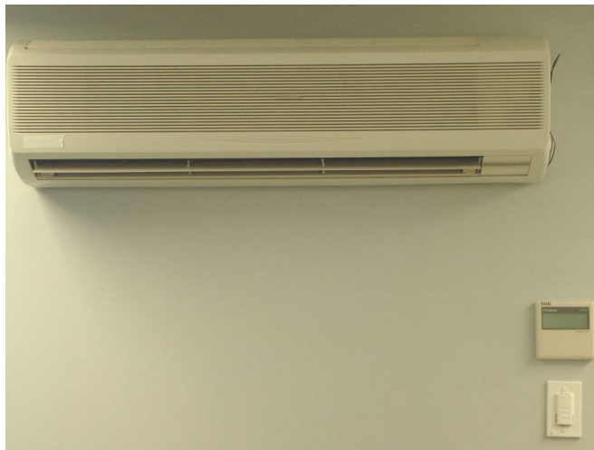
Figure 4.22 : Measurement location under the indoor unit
