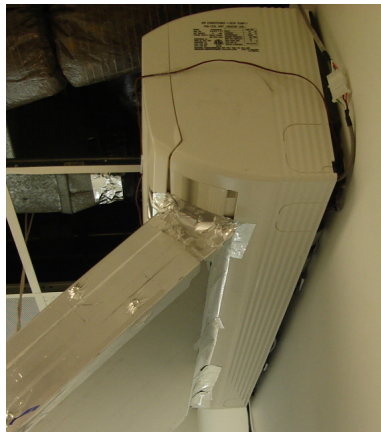
Figure B.2 : Duct taping for the air leakage
