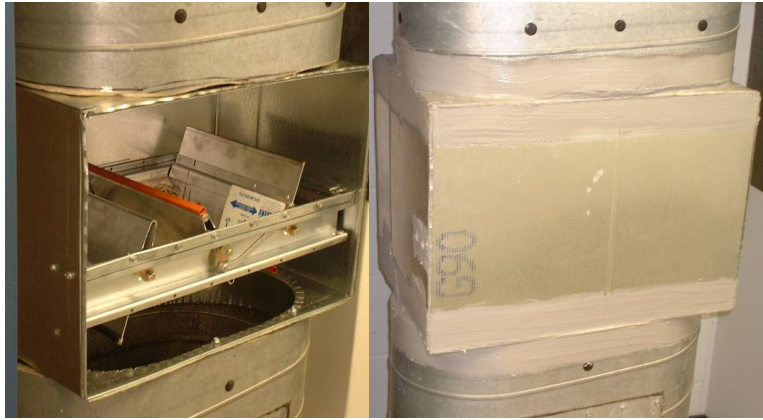
Figure 4.19 : Air damper for supply duct of the existing cooling system
