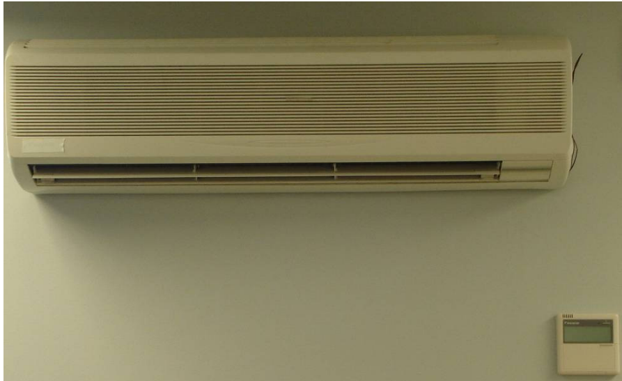
Figure 4.10 : Thermostat and indoor unit
