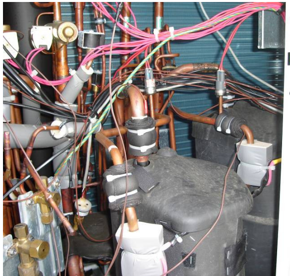
Figure 4.31 : Measurement locations for the compressor refrigerant discharge and suction temperature
