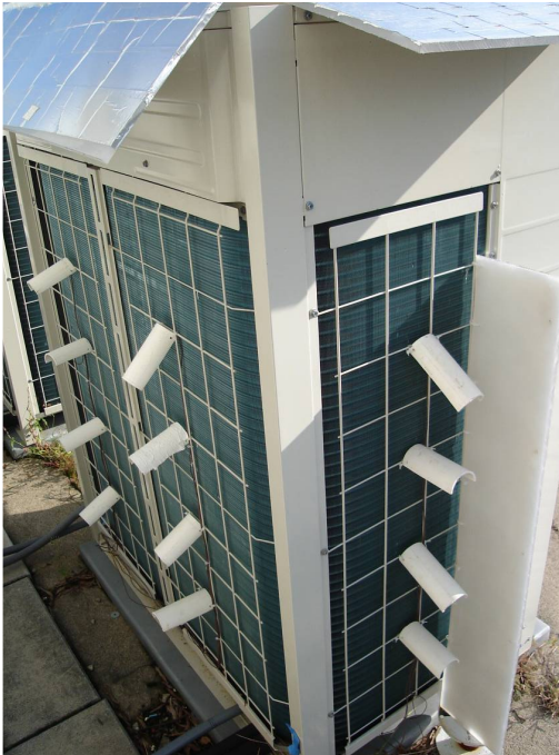
Figure 4.27 : Thermocouple grid around the outdoor unit heat exchanger
