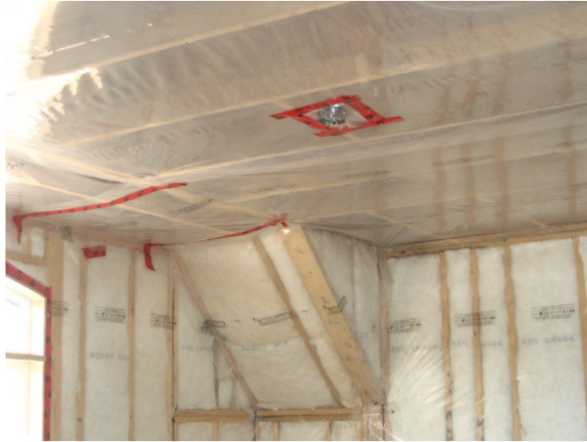
Figure 4-14: Batt Insulation and Vapor Barrier on walls and vapor barrier on the ceiling
