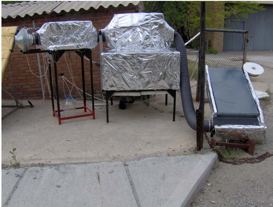
Figure 4.2 A view of the system with insulation
